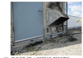
A1 DOOR FLASHING PHOTO
