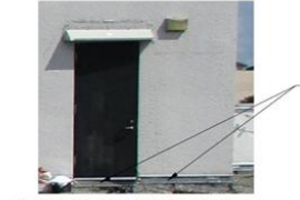
B1 DOOR FLASHING PHOTO
