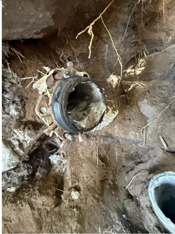
Figure 5: Existing fire service
