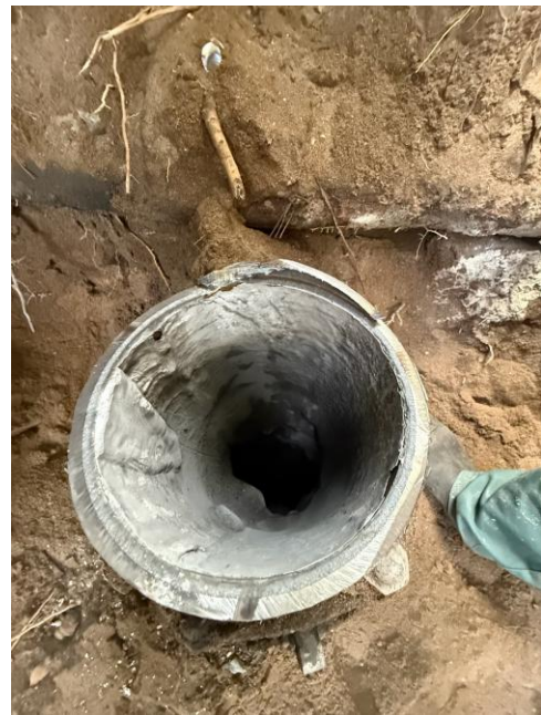
Figure 4: Existing fire service
