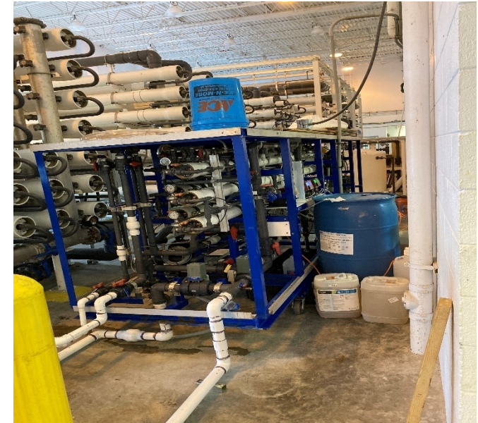
Nanofiltration Membranes at the West plant
