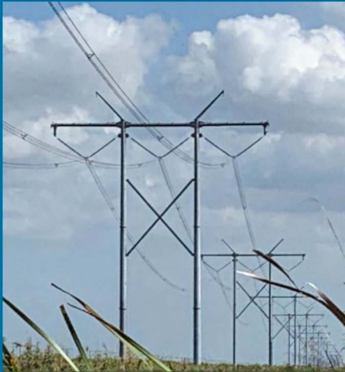
Transmission and substations
