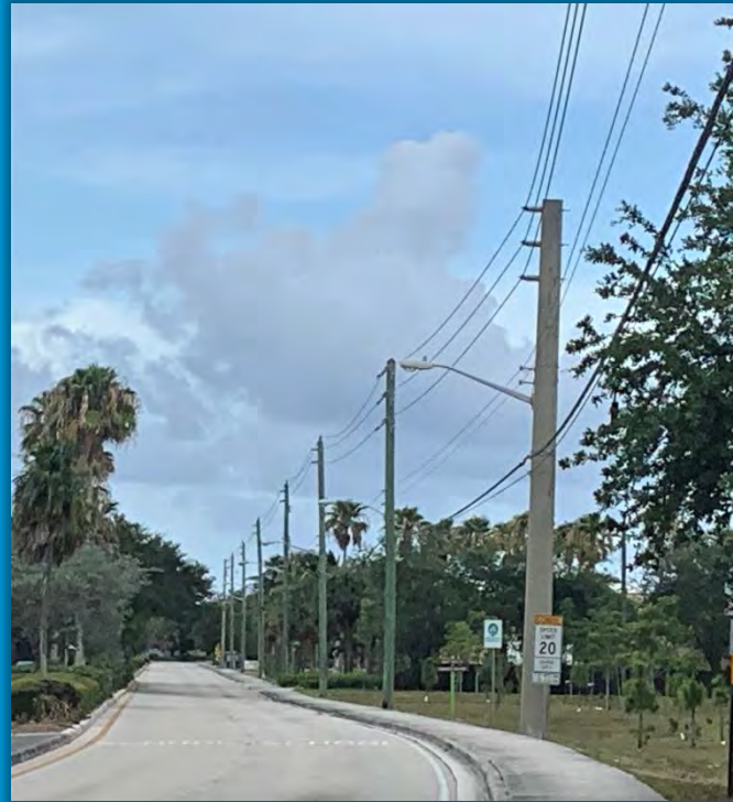
Distribution “feeder” lines
