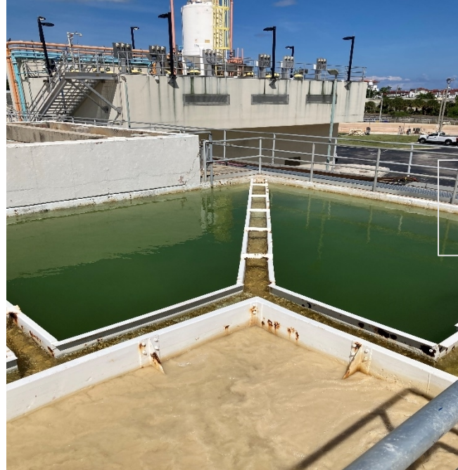
Sedimentation and Filtration at the East Plant
