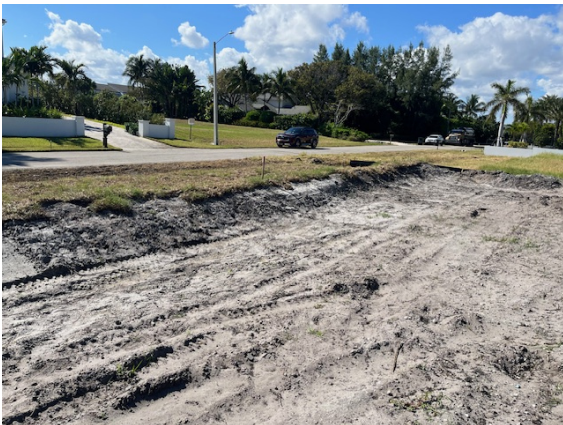
Back of berm-dirt sloughing
