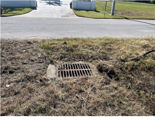
Loose dirt around catch basin
