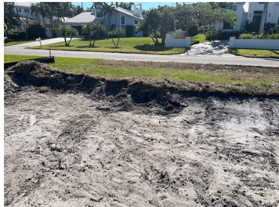
Back of berm-no erosion control
