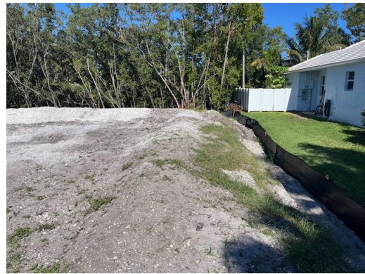
No erosion control
