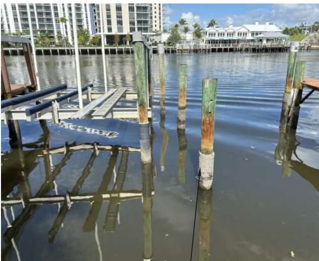
PILE CONDITION UNDERNEATH THE CONCRETE JACKETS ARE LIKELY BAD.
