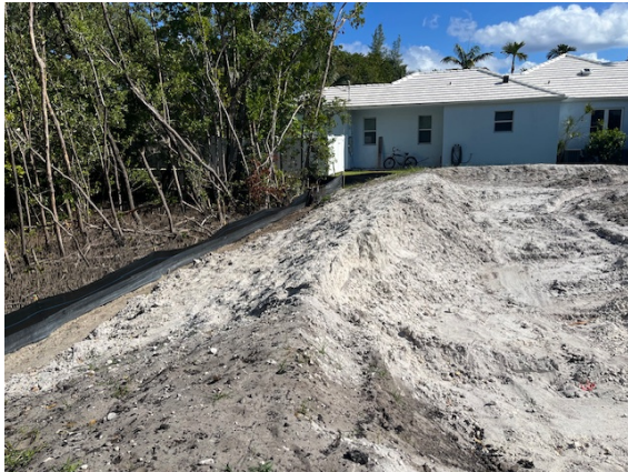
No erosion control
