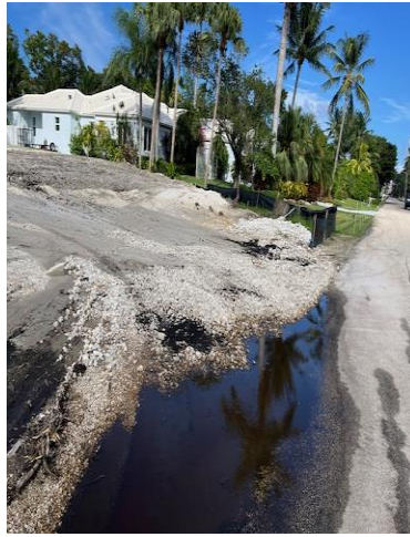
Dirt/debris in ROW
