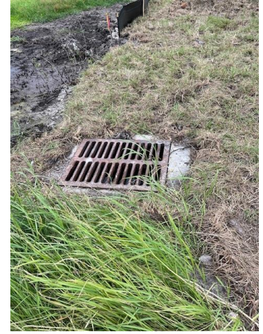
Hudson Ave catch basin
