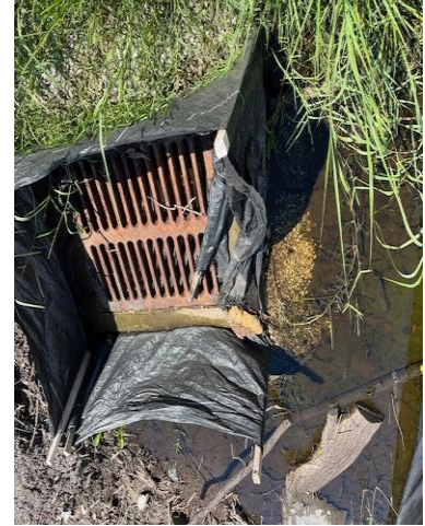
Hudson Ave catch basin
