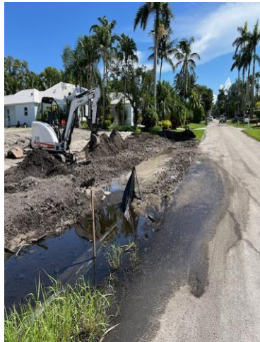
Looking east- debris in right-of way
