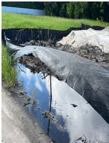
Ponding water within the ROW
