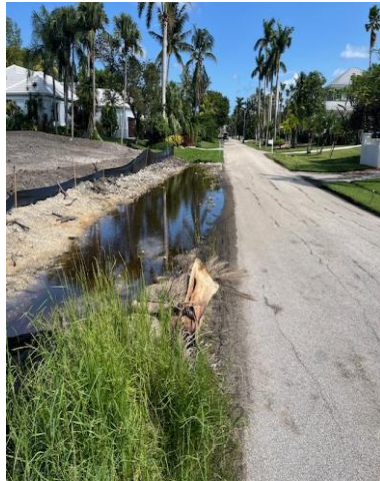
Swale not graded in right-of-way
