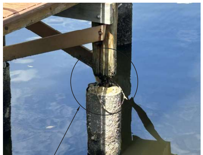
SEVERELY DAMAGED PILE AND CONSIDERED UNSAFE
