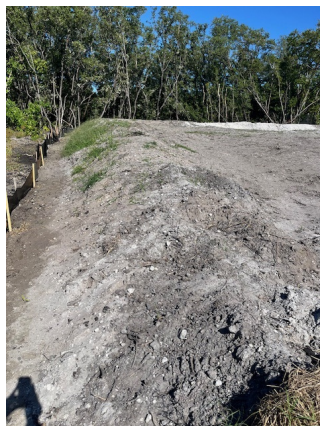
No erosion control
