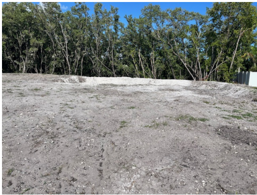
New dirt on berm- no erosion control
