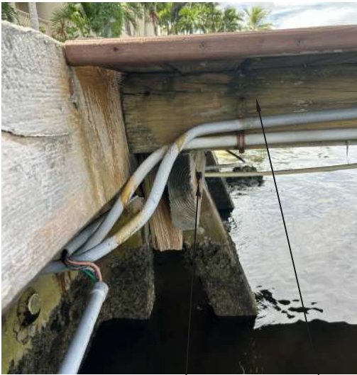
WEATHERED SUPPORT FRAMING CORRODED HARDWARE. MUCH OF THE HARDWARE IS SIGNIFICANTLY CORRODED.
