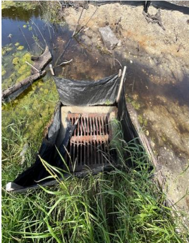
Right-of-way catch basin
