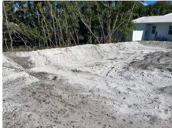
White colored fill-no erosion control
