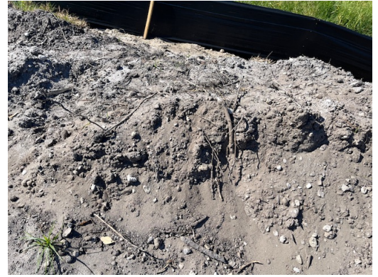
No seed/sod on berm
