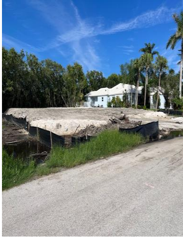
Fill beyond the property line
