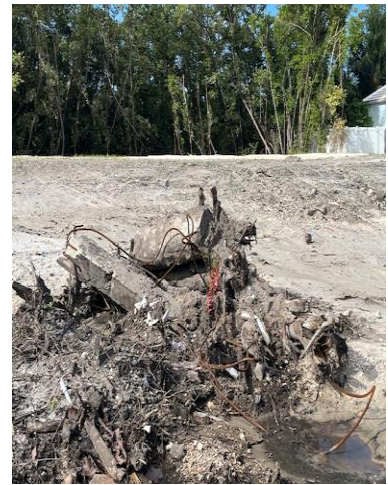
Debris pile at the ROW line
